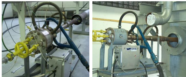
Figure 4. A burner for pulse combustion cooled by water with mounted measuring equipment and connected to the pipe for exhausting flue gases into the environment - left, i.e. applied to the side of the boiler model in the combustion zone - right; Pulse Combustion Laboratory, University of Sarajevo - Faculty of Mechanical Engineering, [28], [35].
