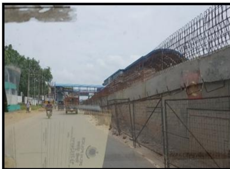
Figure 6 Barricading of working area causing hazard
