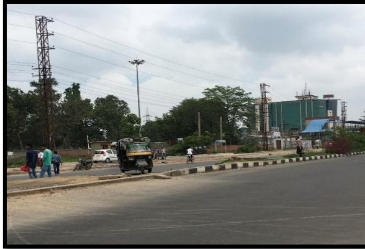
Figure 7 Vehicles climbing over the median due to damaged median.
