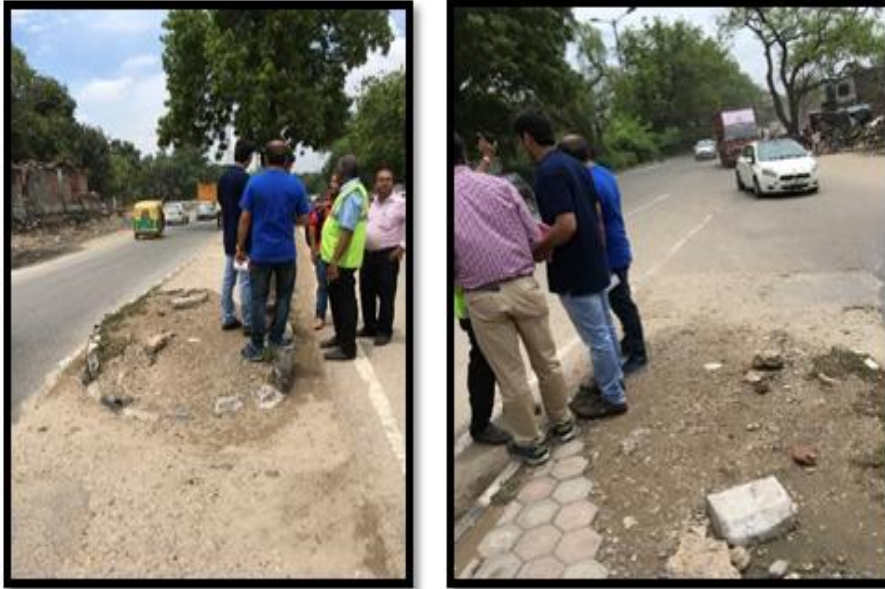
Figure 9 median without sign board and no acceleration lane
