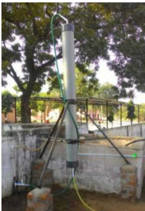
Scrubber for biogas purification
